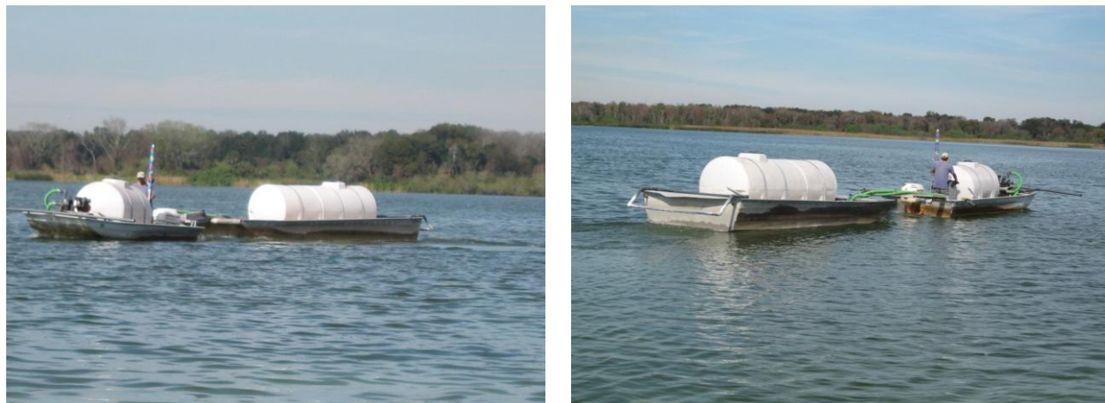
Figure 2-5. Application Boat and Tanker Barge Used for Alum Application in Lake Holden.
